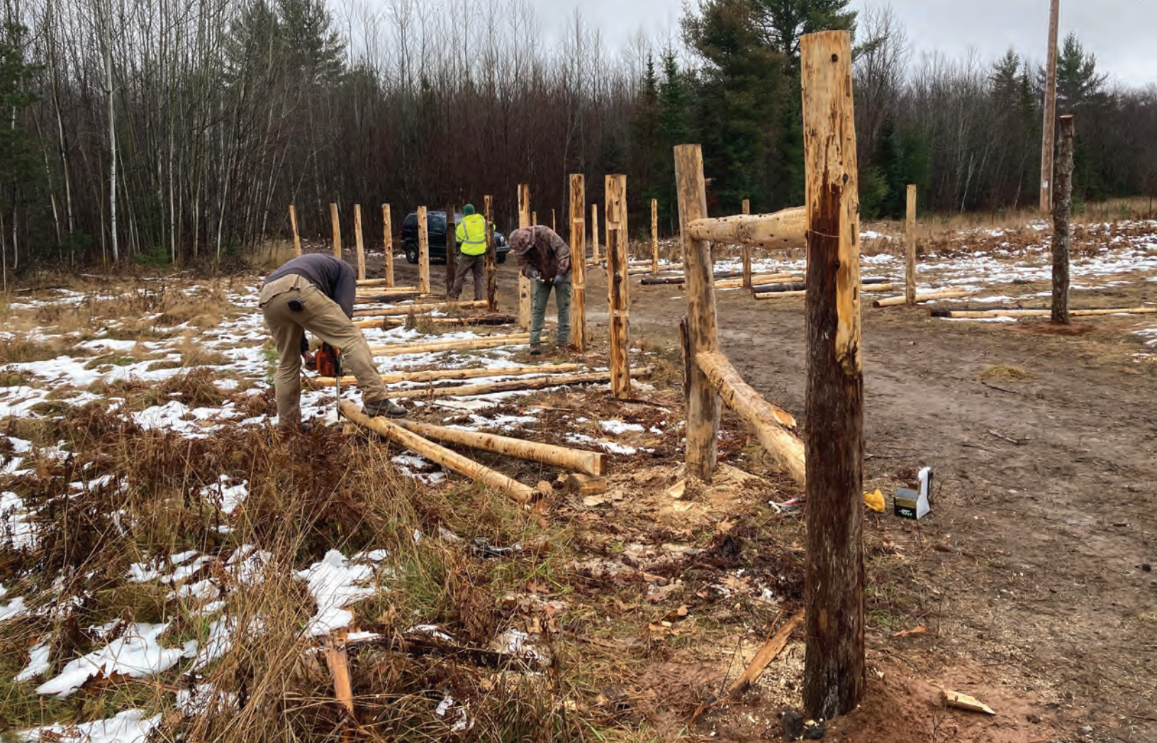
UPLC volunteers work to install a fence that will direct traffic to the new parking area at the Vielmetti-Peters Reserve. UPPER PENINSULA LAND CONSERVANCY
